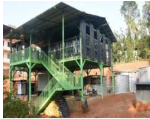
1 MLD STP at Kozhikode medical College
