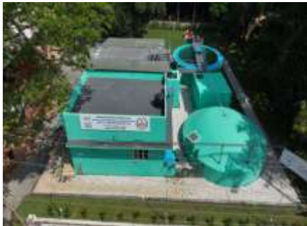
360 KLD STP at General Hospital, Thrissur
