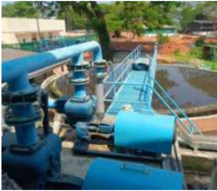
500 KLD STP at Kozhikode medical College
